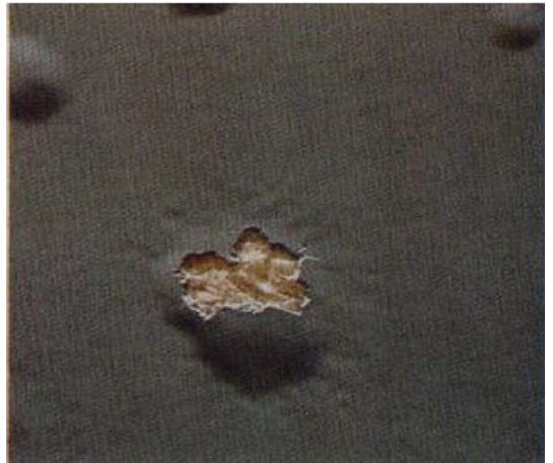
4. Blisters (Caused by catalyst drop)
